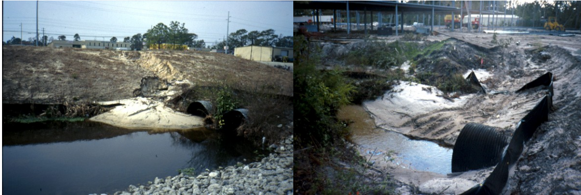
Figure 3. Failing sediment fences in New Hanover County, N.C.
