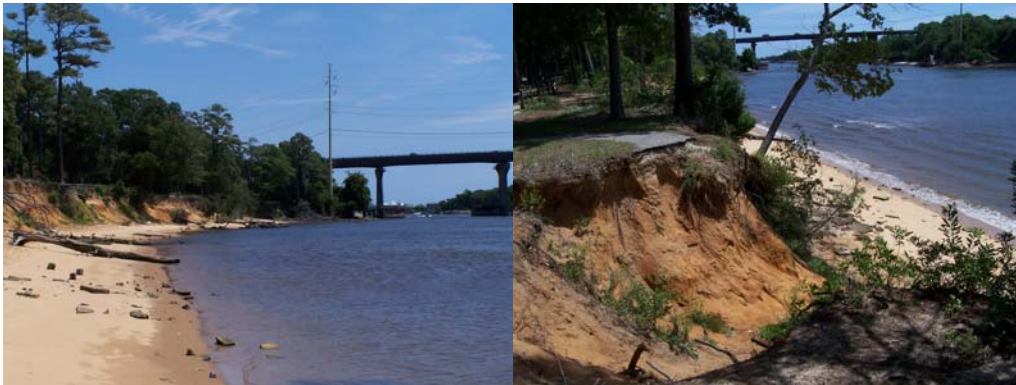
Figure 4. Severe upstream and downstream erosion and bank undercutting of riparian shoreline caused by rerouting of tidal energy away from bridge abutment armored by concrete, Snow’s Cut in the Cape Fear River system, N.C.
